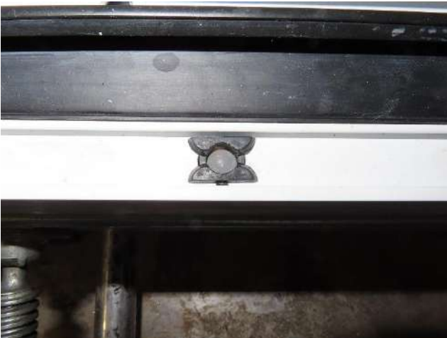
Picture 29 Drainage valve
