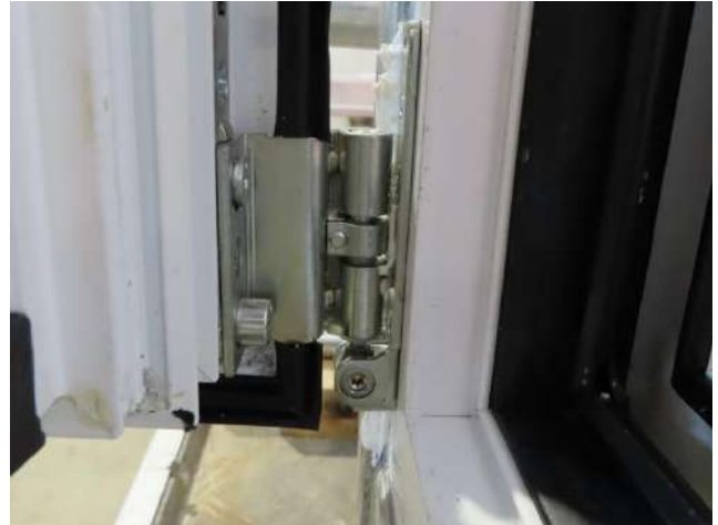
Picture 10 Hinge rebate view, inactive casement at bottom
