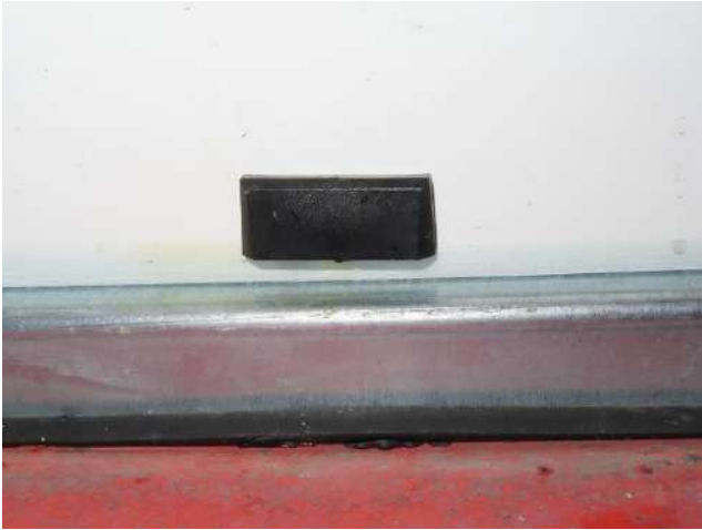
Picture 31 Drainage slot with cover cap, seen from outside
